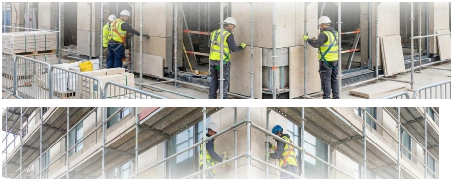
Figure 7. On Site Installation of Stone Panels Using the Mechanical Supporting System (Anchors and L-Brackets) and Alignment Checks
